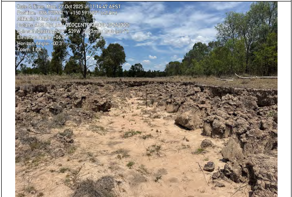
Photo 2: Natural drainage with active erosion zone at the crossing point
