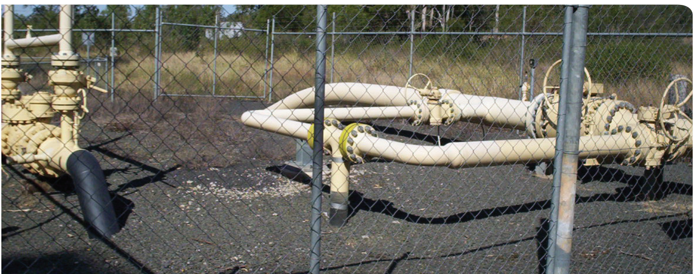
➤ Typical enclosure around a valve on a rural property
